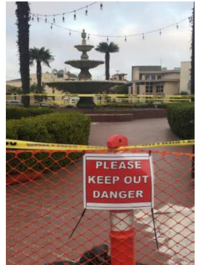
The park walkway tile replacement project was put on hold just days after construction began.
